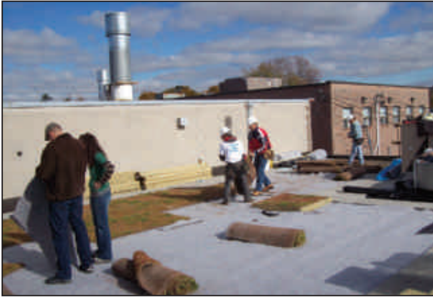
A polyethylene barrier is laid and a fleece layer for water retention.
